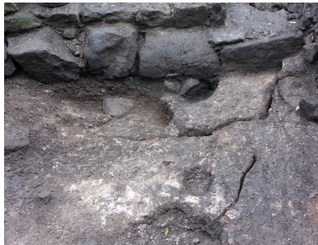
Fig.5 : Attempt to underpin the cross wing.
